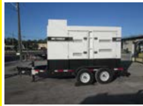
'19 Multiquip 175KW Trailer Mounted Generator - just serviced, ONLY 1800 hours. $59,995.
